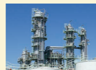
Present tall oil distillation plant
