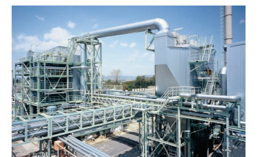
Biomass Power Plant
